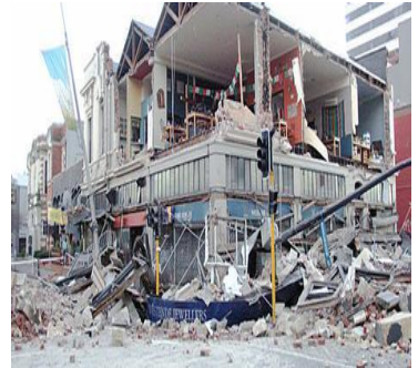
New Zealand Earthquake
